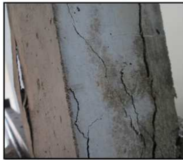
Figure 7: Crack Pattern for Axial Eccentric Loading
